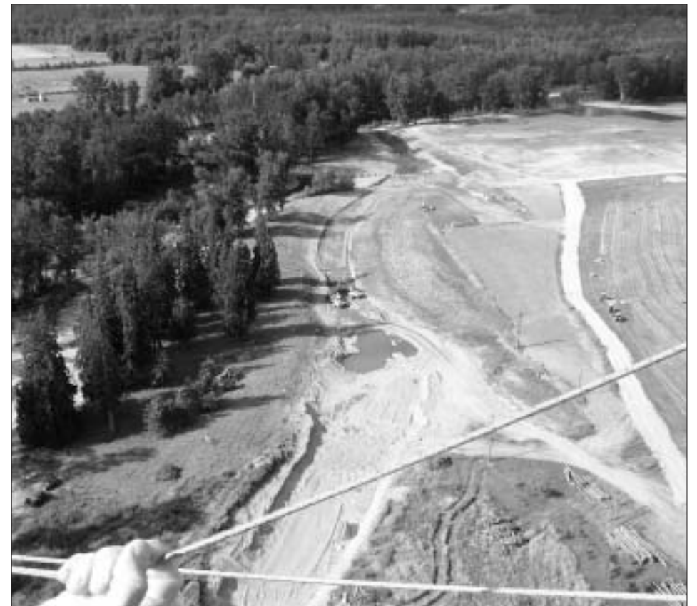
HEAVY EQUIPMENT will remove more than a million cubic yards of gravel from this property, recreating historic river channels that will serve as habitat for salmon fry and other species. Remlinger and Davison hope they will find enough developers to pay them to offset the environmental impacts of development so that they can turn a profit on the restoration of their land. This bird's eye view is from Remlinger's ultralight airplane. PHOTO BY POLLY KEARY
